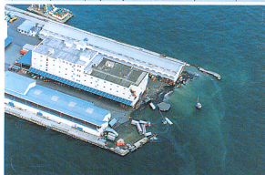
Damaged pier in Kobe Harbor (by Asia Air Survey)
