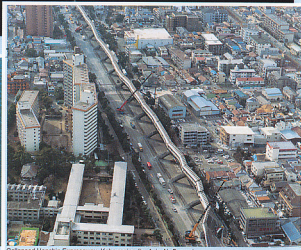
Collapsed Hanshin Expressway, Kobe region (by Asia Air Survey)
