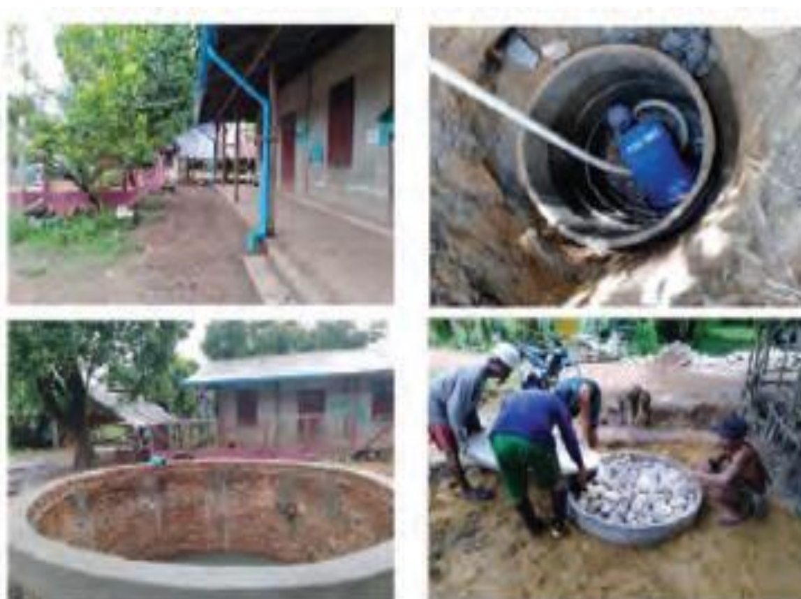
Fig. 6. Photographs of artificial groundwater recharge well in Mawlamyine, Mon State
