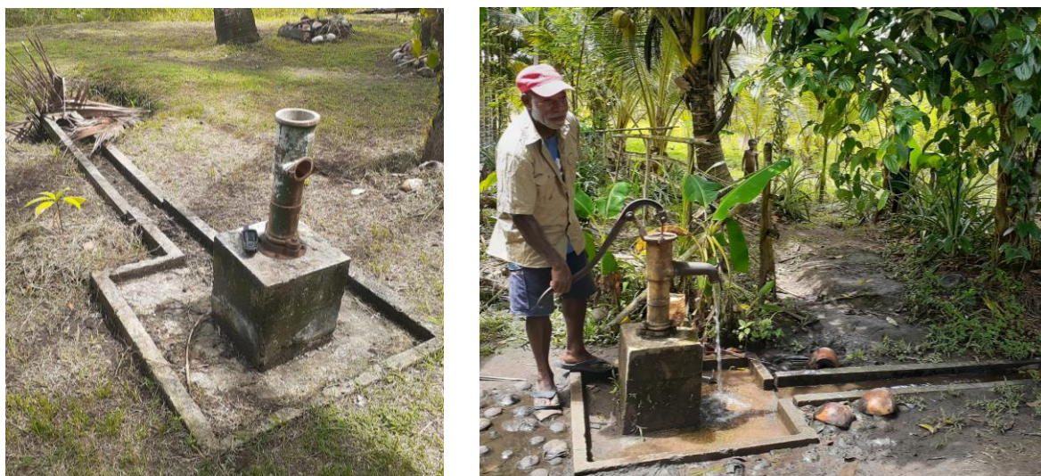
Fig. 3. A dysfunctional hand pump (left) and a currently functioning hand pump with the caretaker (right) in Giringarede village, South Fly District, Western Province
